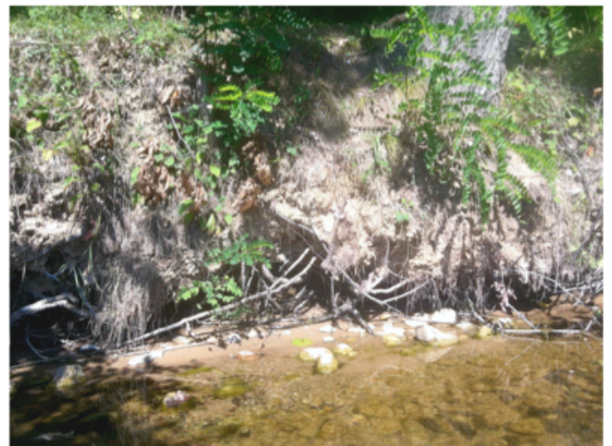
Photo 1 [Typical undercut along Section A]
