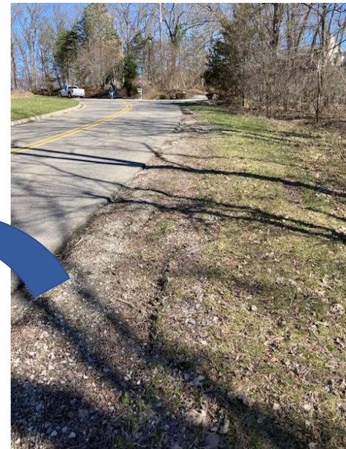
Issue: erosion of berm, potential for undercutting the road
