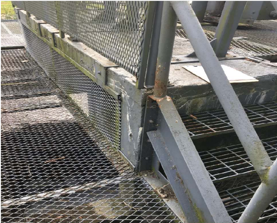
RUSTING & DETERIORATION ON STEEL SURFACES OF DAM CONTROL STRUCTURE
