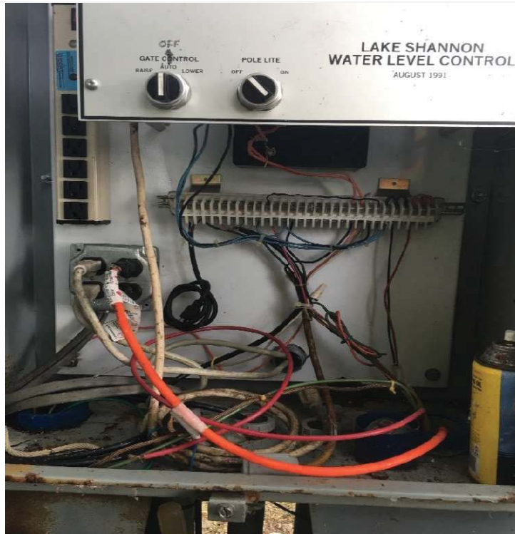
WATER LEVEL CONTROL ELECTRICAL BOX OFF DAM CONTROL STRUCTURE
