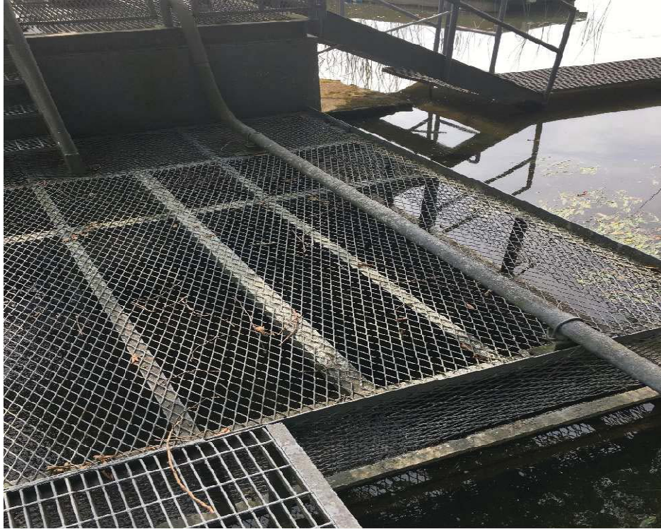
ELECTRICAL CONDUIT- ELECTRICAL BOX TO THE DAM CONTROL STRUCTURE
