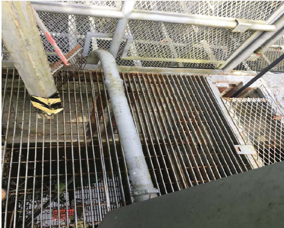
CLOSE UP OF ELECTRICAL CONDUIT AS TRIP HAZARD
