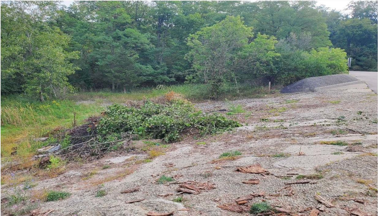
NORTH EMBANKMENT OF EMERGENCY SPILLWAY LOOKING EAST, DEBRIS PILE IN MIDDLE OF CONCRETE SLOPING SURFACES
