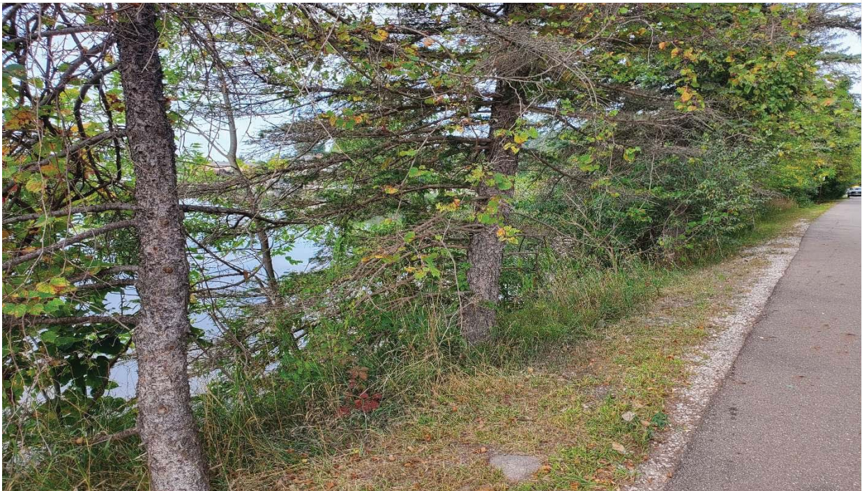
TYPICAL TREE AND BRUSH GROWTH BUILDUP ON THE SOUTH EMBANKMENT
