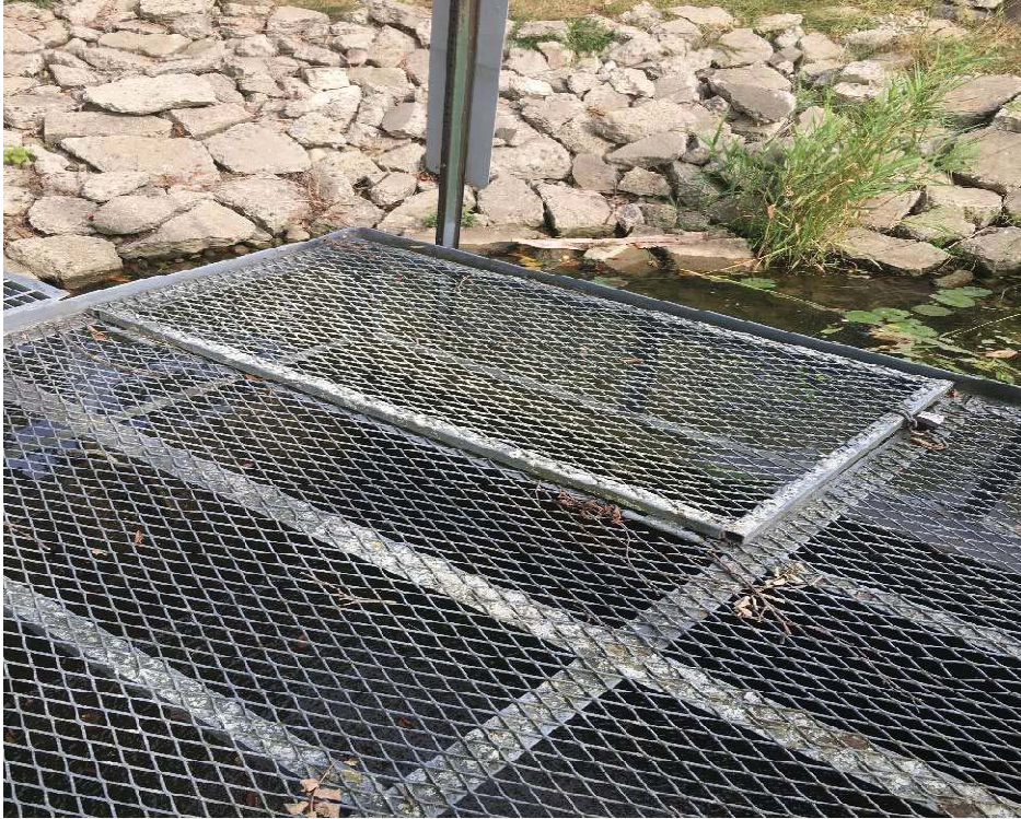
TRIP HAZARD ON DAM CONTROL STRUCTURE
