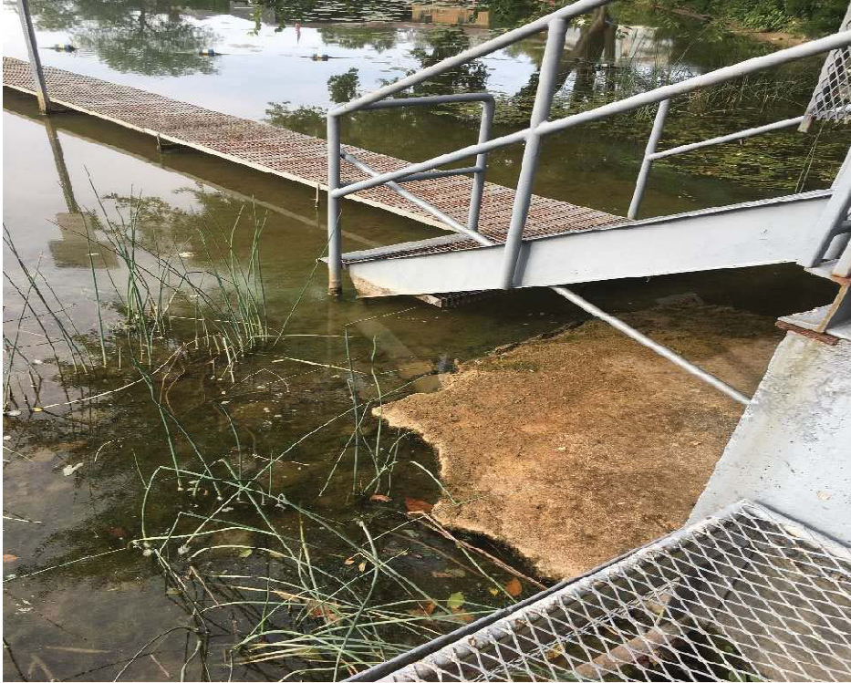
SEDIMENT BUILDUP, SOUTH SIDE OF DAM CONTROL STRUCTURE
