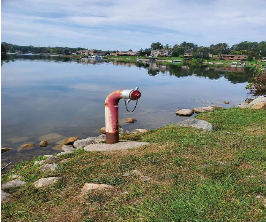
EMERGENCY DRY HYDRANT VALVE
