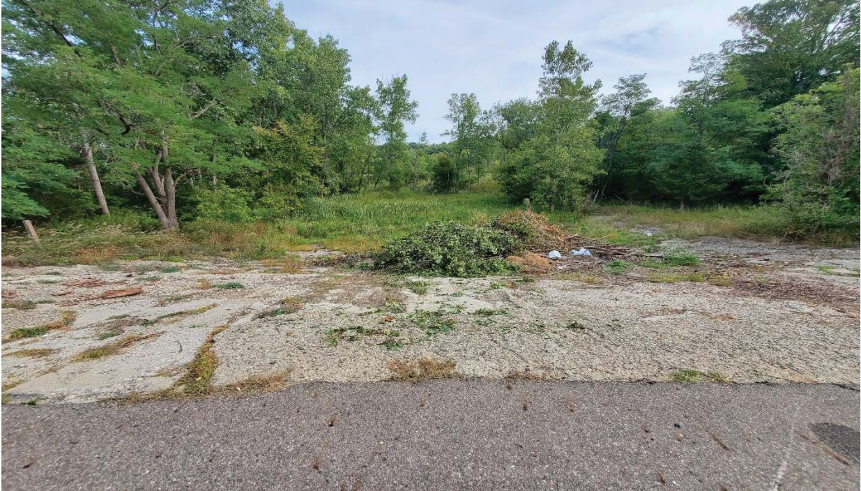
NORTH EMBANKMENT OF EMERGENCY SPILLWAY LOOKING NORTH, DEBRIS PILE BUILDUP IN MIDDLE OF CONCRETE SLOPING SURFACES
