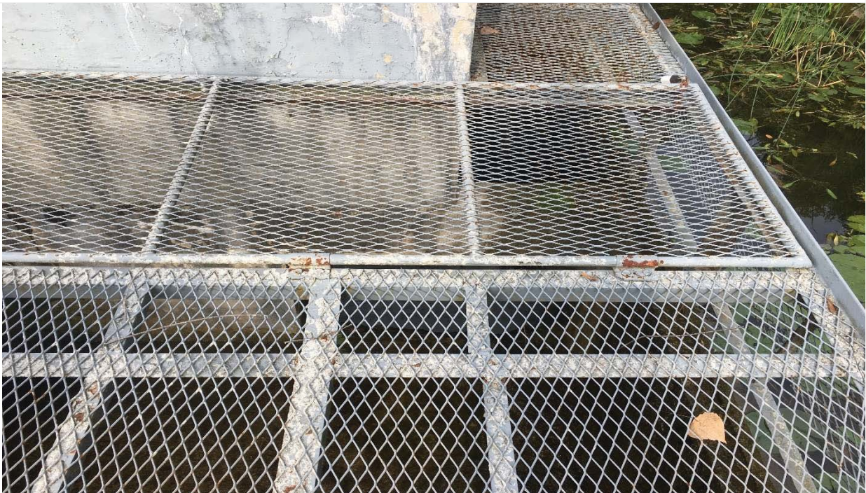
TRIP HAZARD ON DAM CONTROL STRUCTURE
